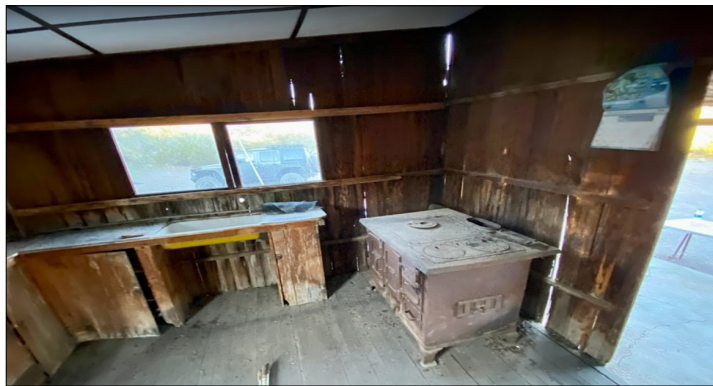
The wood burning kitchen stove that is still present today Jack had brought into the cabin from one of the abandoned mines and placed it in the corner before the walls were erected.
